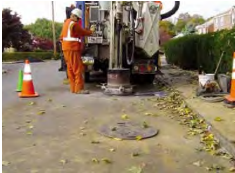
Coring the pavement and using round road plates (foreground) to temporarily cover the excavation
